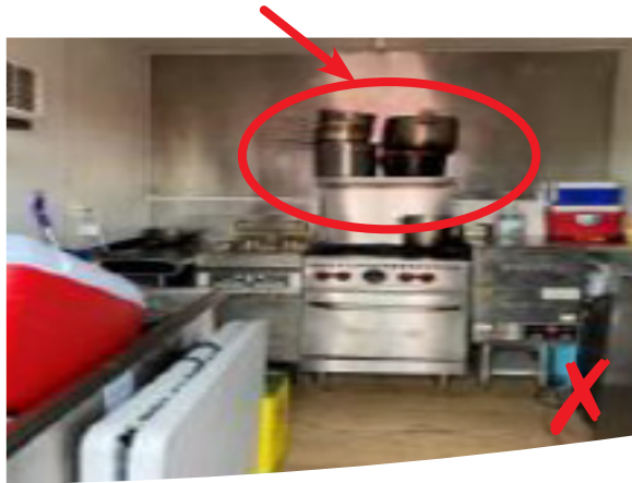
No hood or fire suppression over the installed appliances
