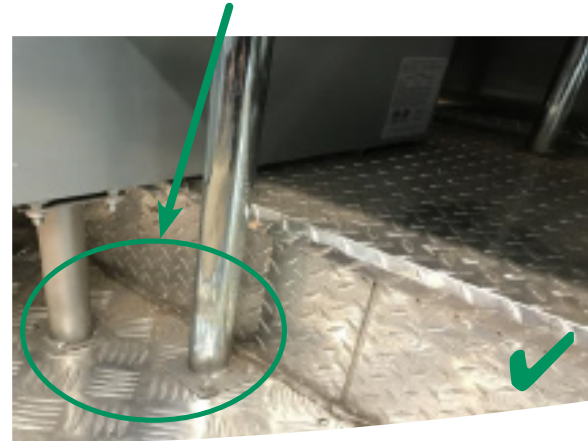
Properly installed and secured to floor per manufacturer's instruction
