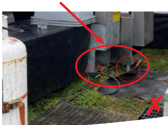
Not installed on a firm and leveled base
