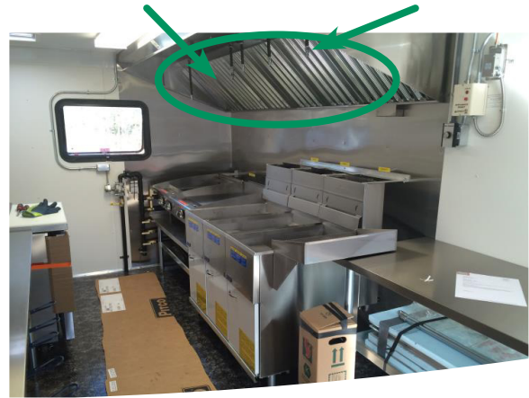
Hood covers appliance Fire suppression installed
